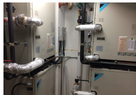
Water-cooled condensing units located in a mechanical room. Internal installation is required for W-VRV condensing units
